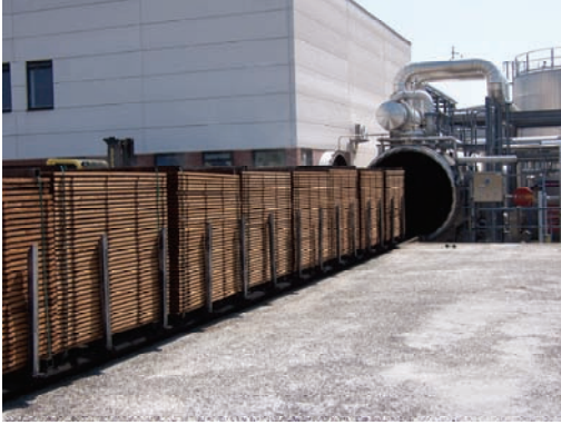
Fig. 1.2 Industrial plant for the hydro-thermolysis stage
