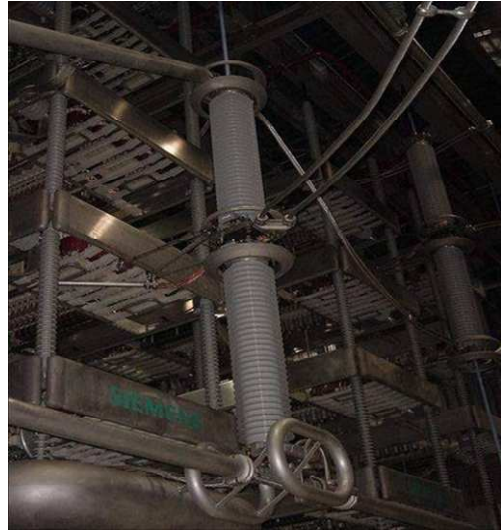
c) Surge arrester
