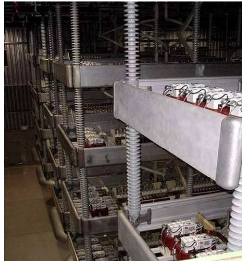
d) Insulator structure
