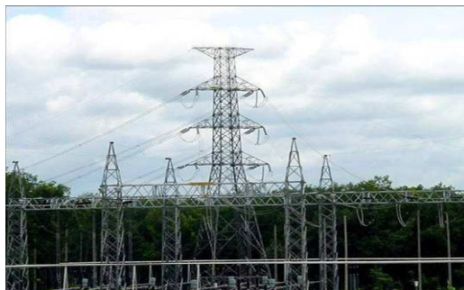
c) 230 kV, AC transmission line
