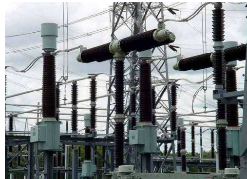
d) Circuits breakers
