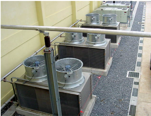
c) Valve cooling system b-Station
