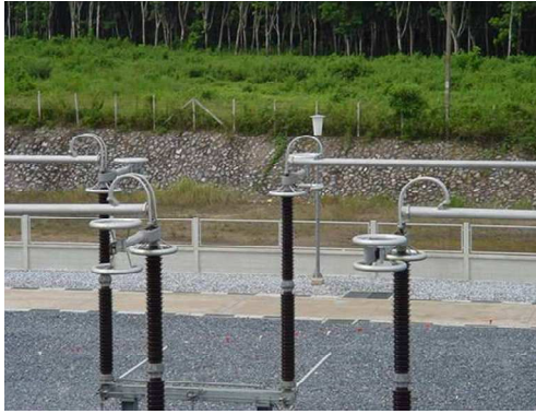
a) Disconnecting switches
