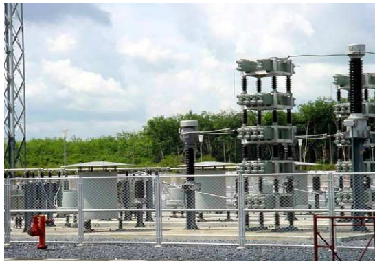
a) AC filters and shunt capacitors
