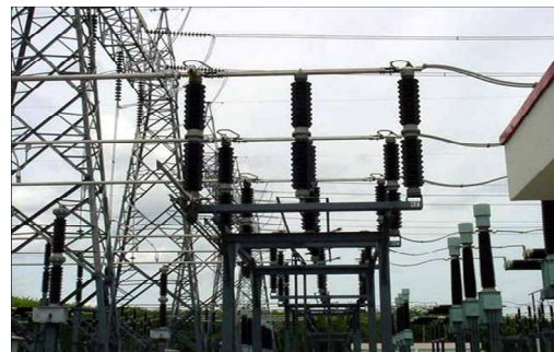
f) Disconnecting switches
