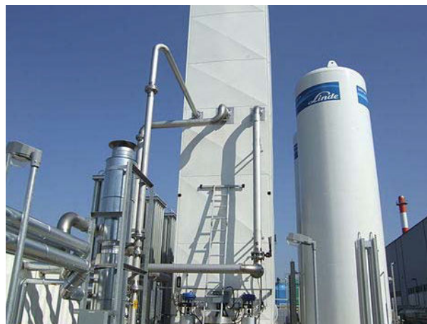
Figure 1.1: Cryogenic distillation industrial plant (Linde company)
