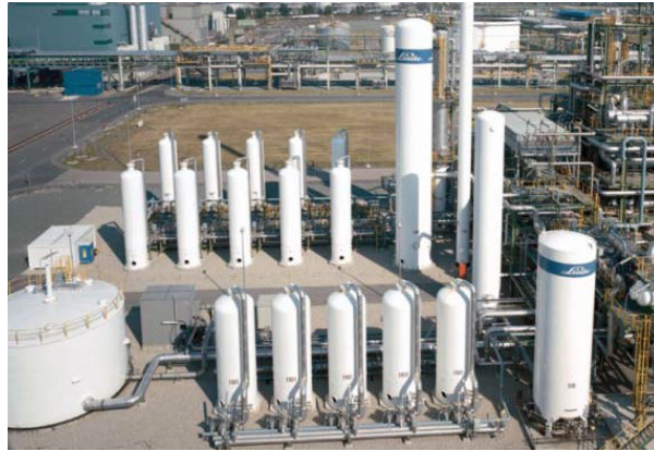
Figure 1.3: PSA industrial plant (Linde company)
