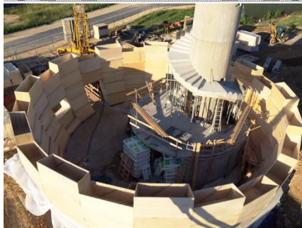
Figure 151. Solar Energy House. Top. Structural members staggered. Notice that the roof rests over the cassette-made enclosing wall. Middle. Closing wall variable section. Bottom. Aerial view of the structure's mounting process. Notice that timber cassettes are installed empty. Insulating material was blown-in once the mounting was finished. Image credits. Top, O.G; Middle, Cartignies-Canonica architects; Bottom, charpentres-bois.com
